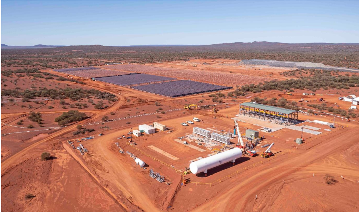
Figure 2 – Work progress on site with the power station & solar farm installation (7 June 2022).
