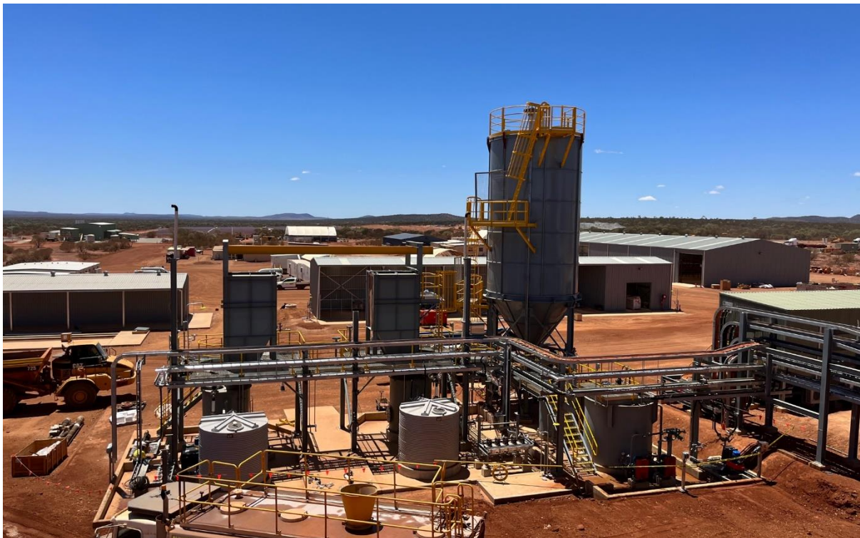
Figure 12 – Plant reagents area with adjacent workshops(right) and laboratory (left) (Photo 11 November).
