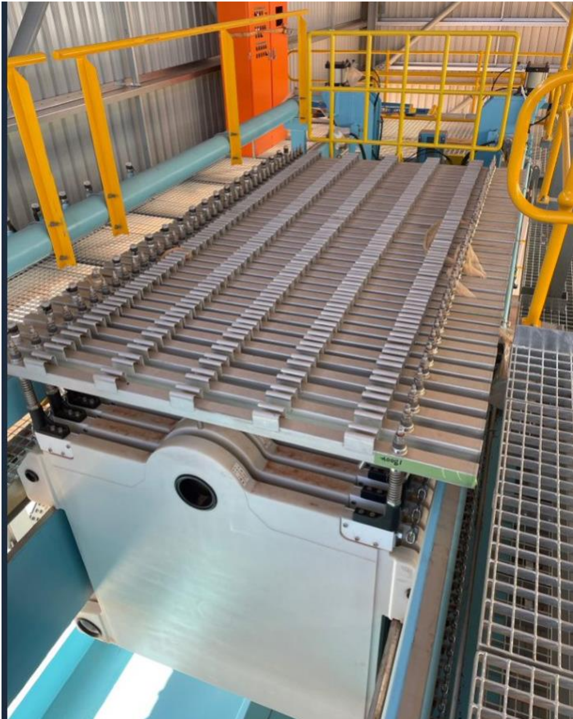
Figure 13 – Concentrate shed filter press.
