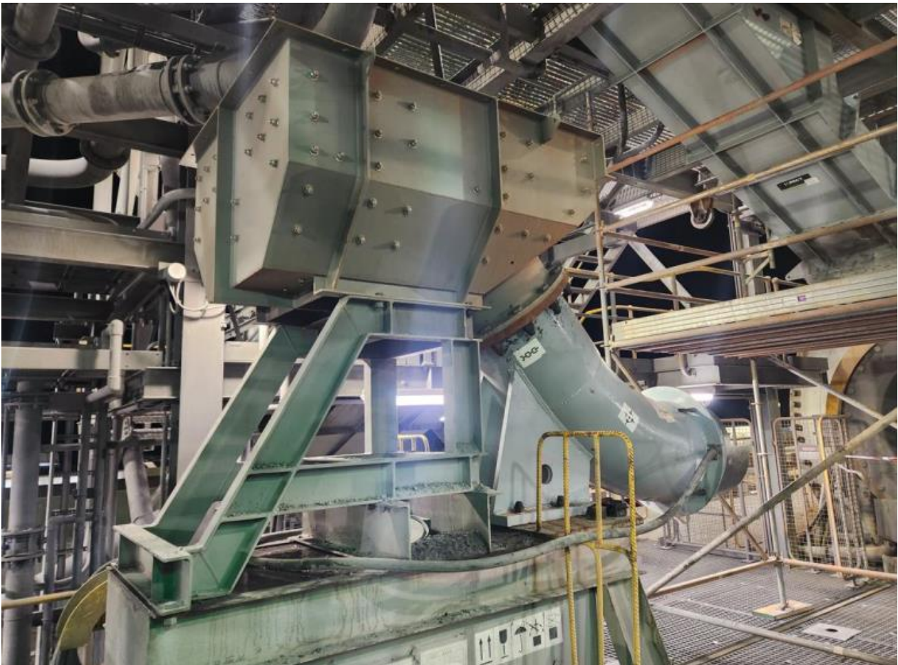
Figure 7 – Picture showing newly maintained mill feed end of the mill (Photo July 2024).
