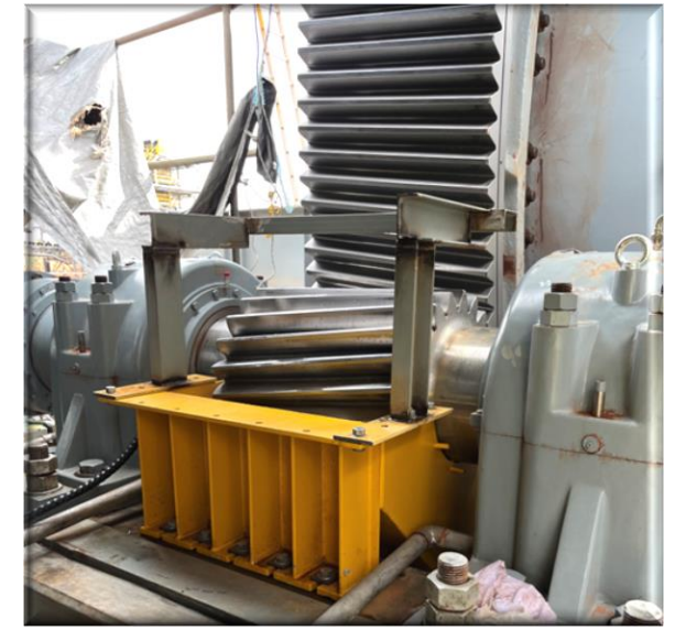
Mill Pinion & Girth Gear
