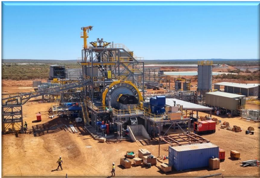
Grinding, Flotation & Filtering Sections
