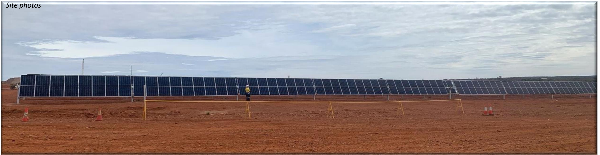
16,000 solar panels fully integrated
