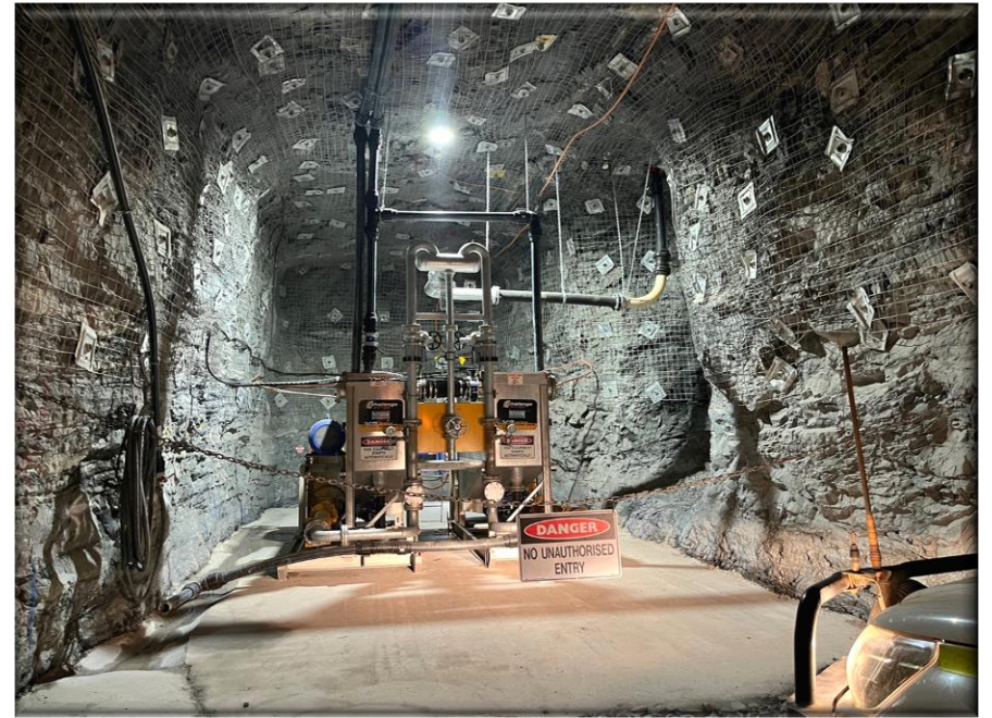
Underground pump station
