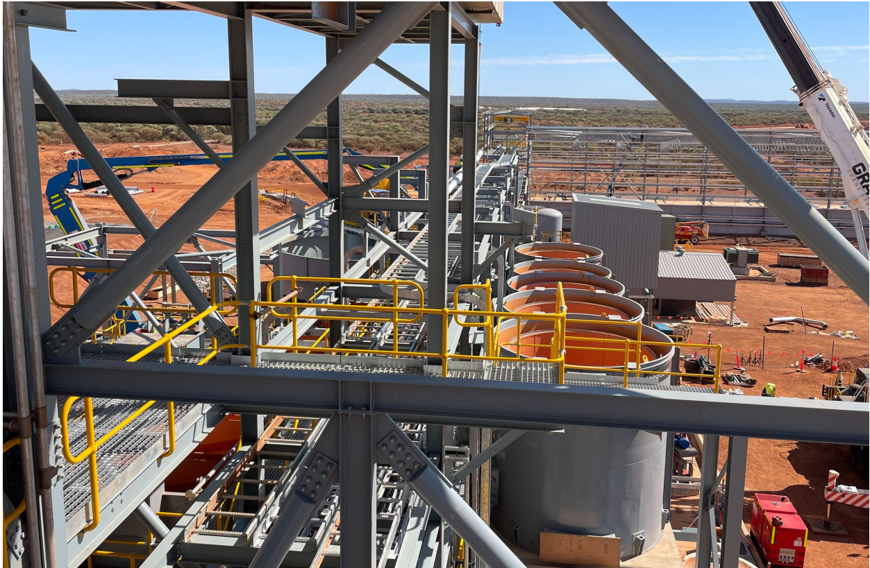
Figure 2 shows the installation of the flotation cells in the Abra processing plant (photo: 22 September 2022)
