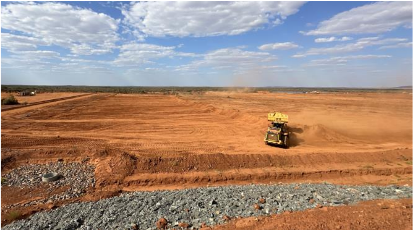
Figure 8 – Picture of tailings storage facility (TSF) cell B under construction (Photo September 2024).
