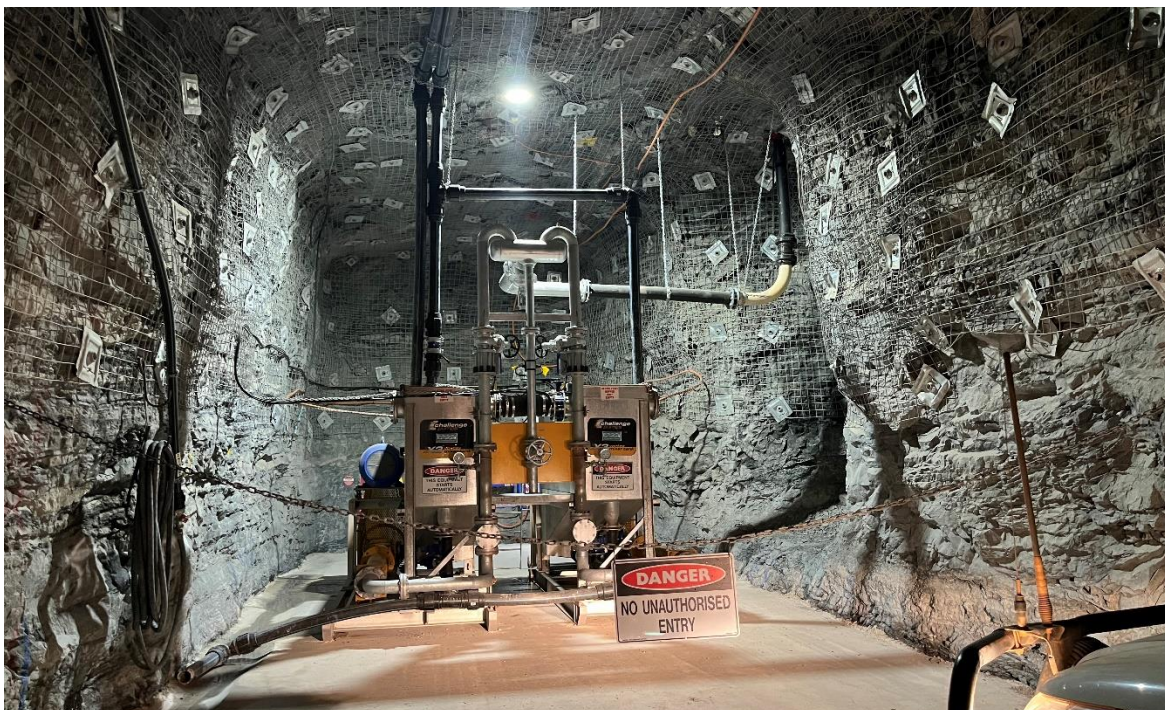
Figure 12. Underground pump station (Photo 30 September 2022).
