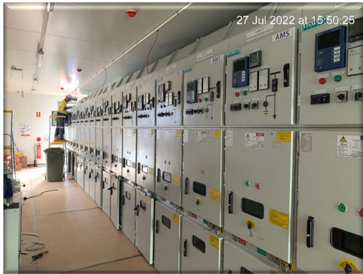
Power Station Switch Room
