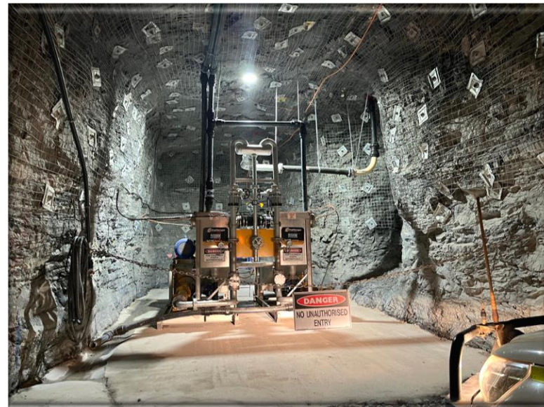
Underground pump station
