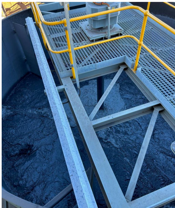
Figure 3 – Concentrate tank filling (photo 3 May)
