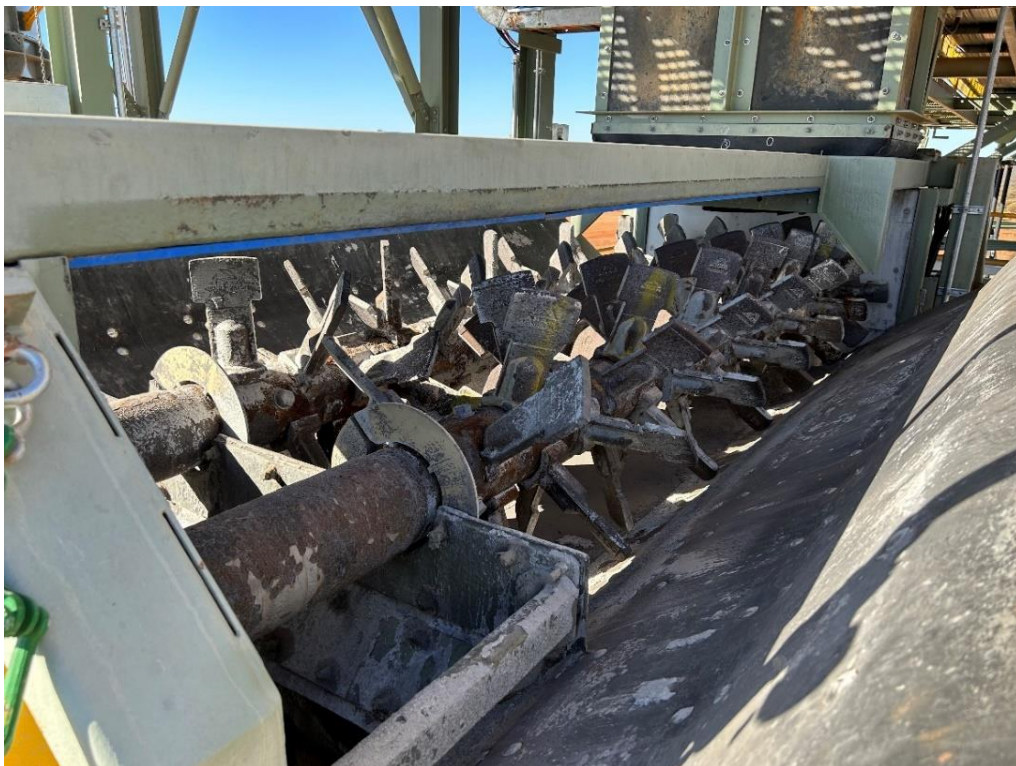
Figure 10 – Internal view of the paste mixer used for mixing paste (tailings and cement and water) at Abra (Photo 5 September 2023).
