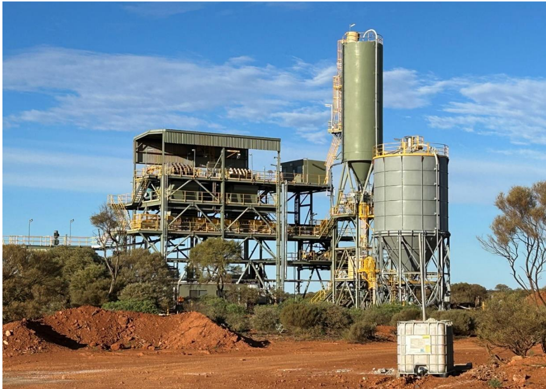
Figure 7 – Abra paste-fill plant.
