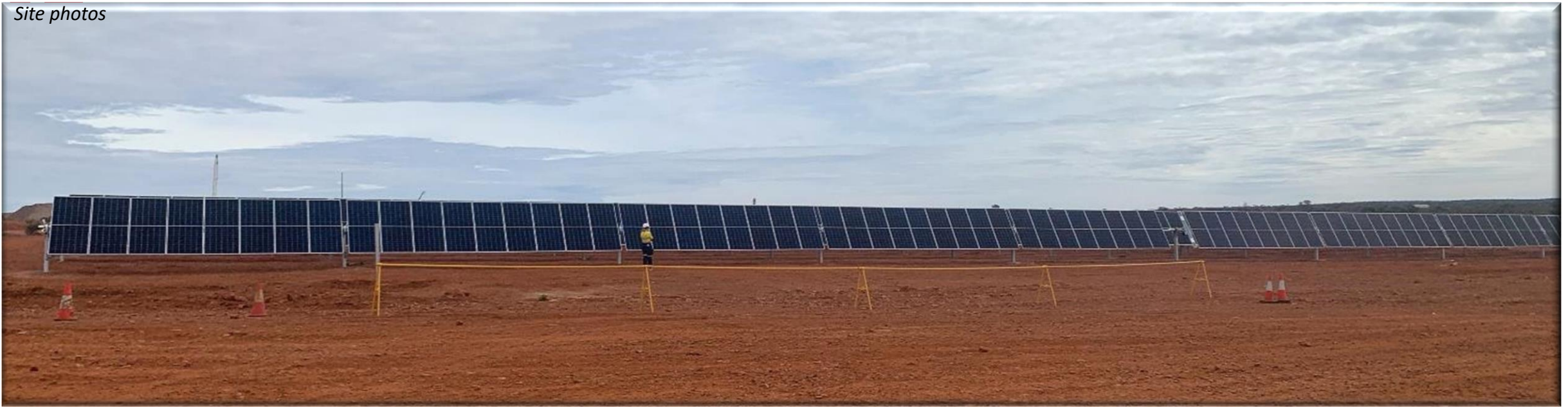
16,000 solar panels fully integrated
